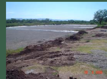
Subsurface non vegetated constructed wetland. August, 2006
